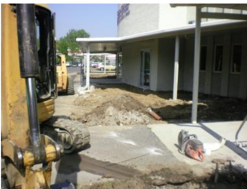
Extensive work to prevent further damage to the corps building began on September 30.
